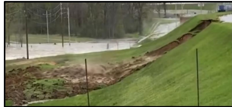
40-second time-lapse of Edenville Dam Breach FEMA Incident Response Review 2022
